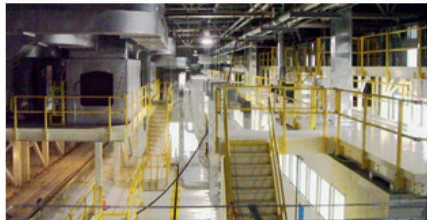
The bumper system is designed with a working area on three levels with a length of 65 meters
